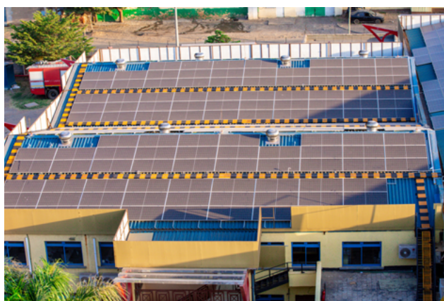
225kWp solar photovoltaic power plant at the KPC HQ
