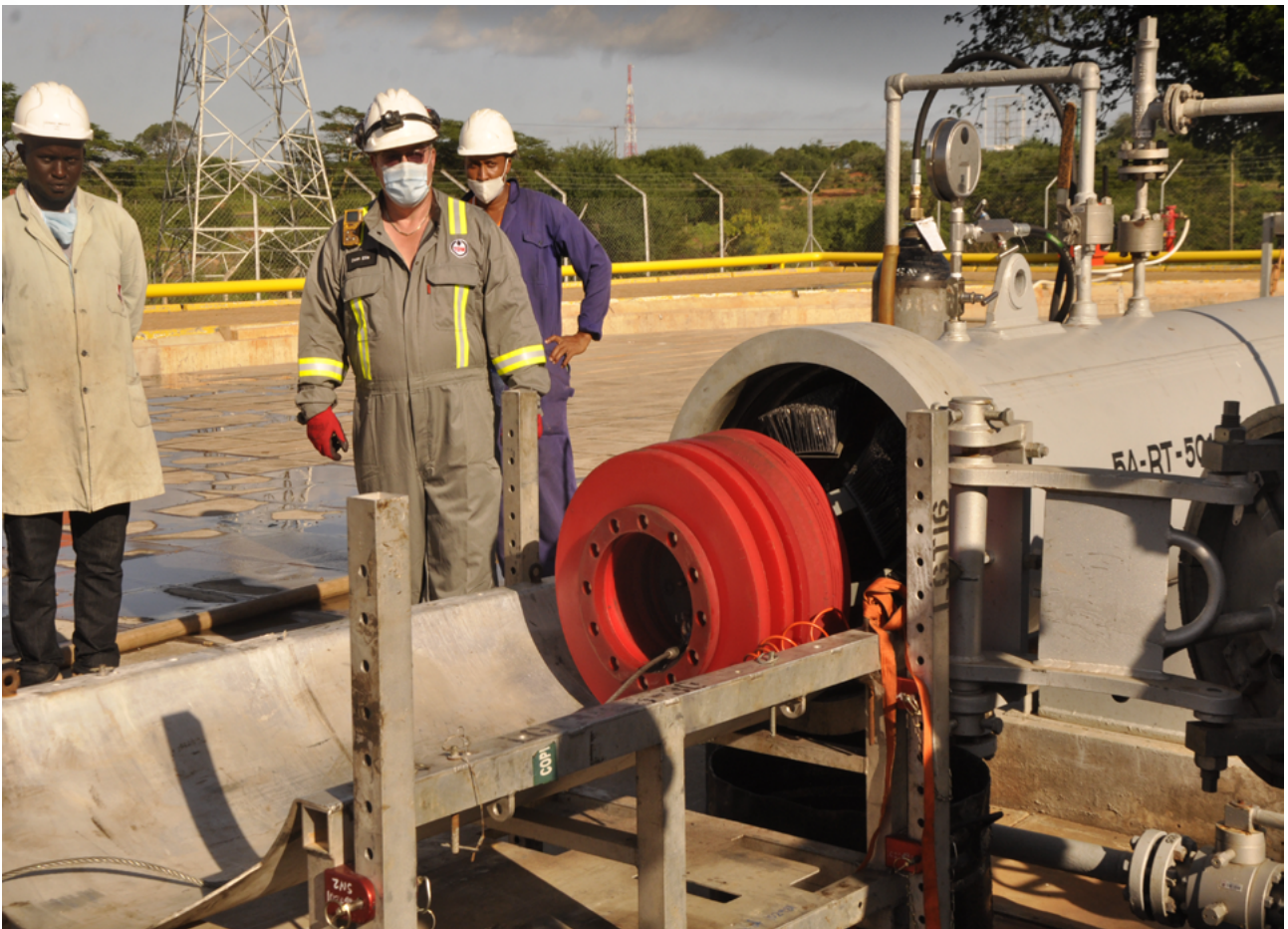
Pipeline inspection (pigging) process at PS 7 to ensure the integrity of the pipeline.
