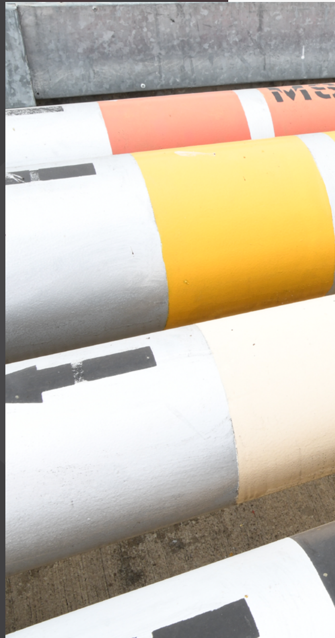
Inter-sites pipelines at Kisumu (PS28) Depot
