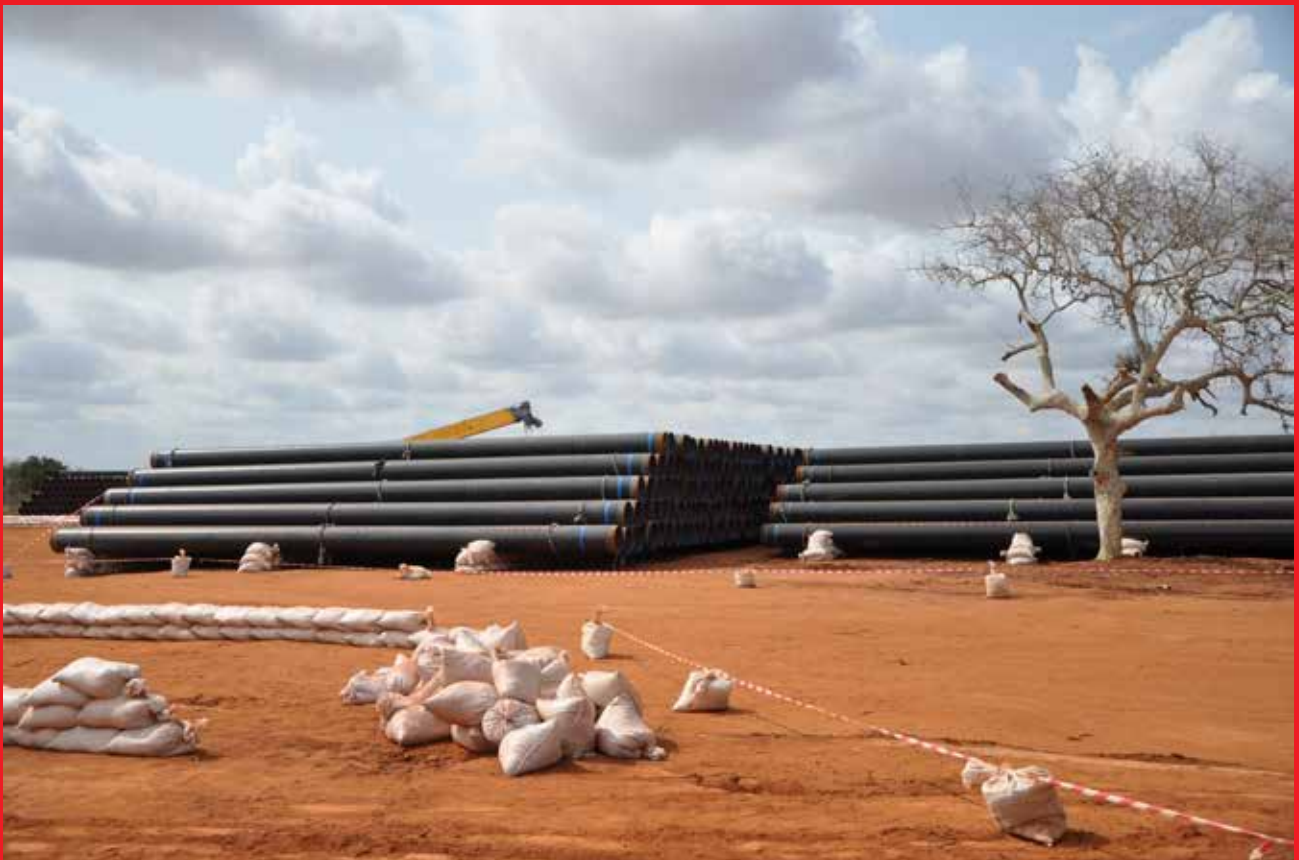
Stock piling of pipes at Pump Station No 5 - Maungu for the Line 1 Replacement Project
