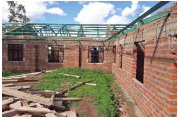
Ongoing construction of administration block and classes at Masangora Girls Secondary School.
